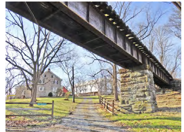
Bridge that carries the Devault Line in Charlestown Township. Image credit: Campbell Thomas and Company.
