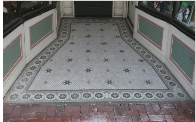
The colors of the paneled wood storefront apron complement the tile colors in the flooring.
