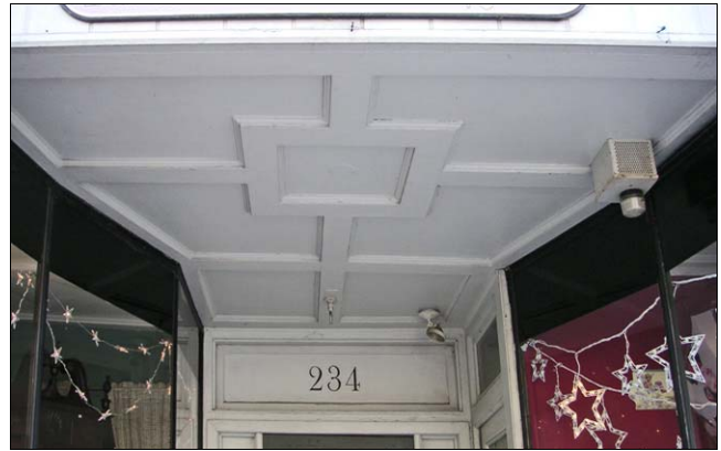
This storefront entrance alcove has an unusual shape that narrows back towards the central entry. The ceiling pattern highlights the geometry of the space.
