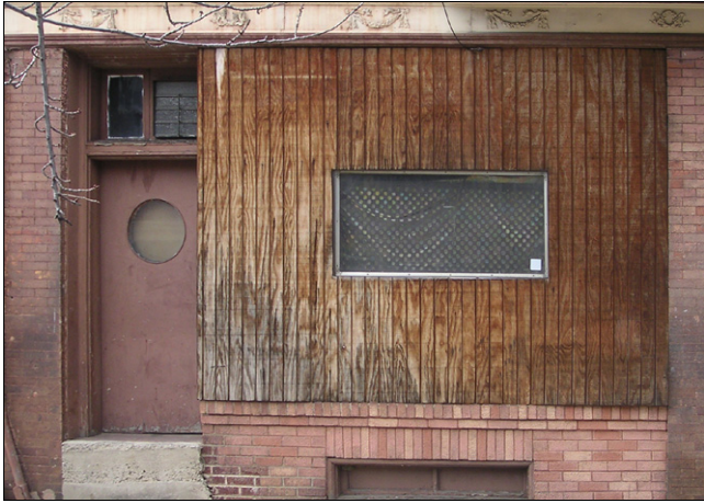
This storefront window has been infilled with wood reducing the window opening size and changing the character of the building.
