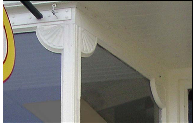
The vertical supports flanking the storefront glazing has quarter-round fan shaped trim that complements the architectural style of the storefront and building.
