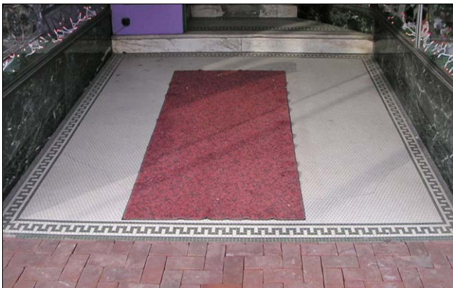
This tiled entrance alcove floor has a solid color center surrounded by a geometric pattern border.
