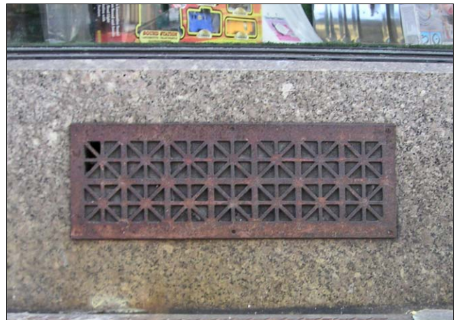
The granite apron provides a base for the storefront window glazing system. The former vent grille is an architectural feature that should be retained.
